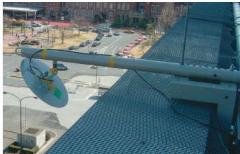
Pseudolite installation on roof for Tsukuba test
